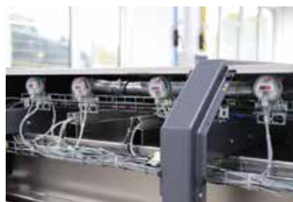
Integrated filter monitoring of the individual zones including volume flow control
